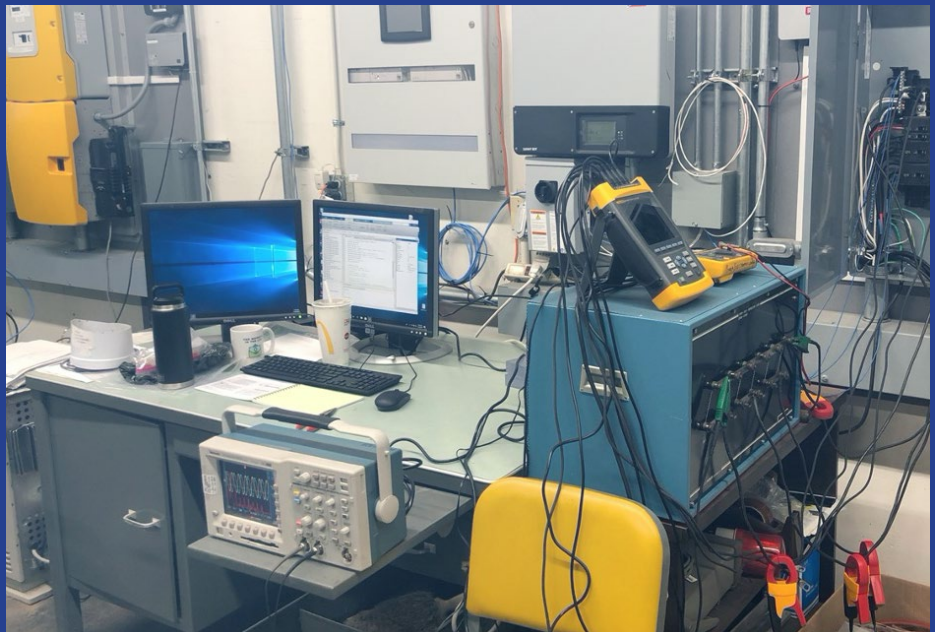
CDR Hirsch's research included a three-phase microgrid set up with three commercial-off-the-shelf (COTS) inverters and a battery bank as its energy storage system.
