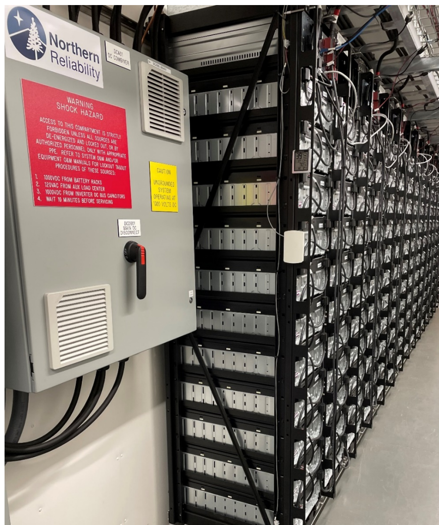
Figure 16: A Battery Energy Storage System at the Microgrid Testbed at NAVFAC EXWC
