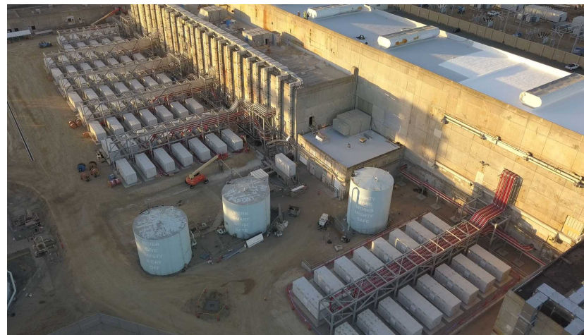
Vistra Energy, Moss Landing, Monterey, CA - 300 MW / 1200 MWh - Peaker Replacement, Grid Reliability
