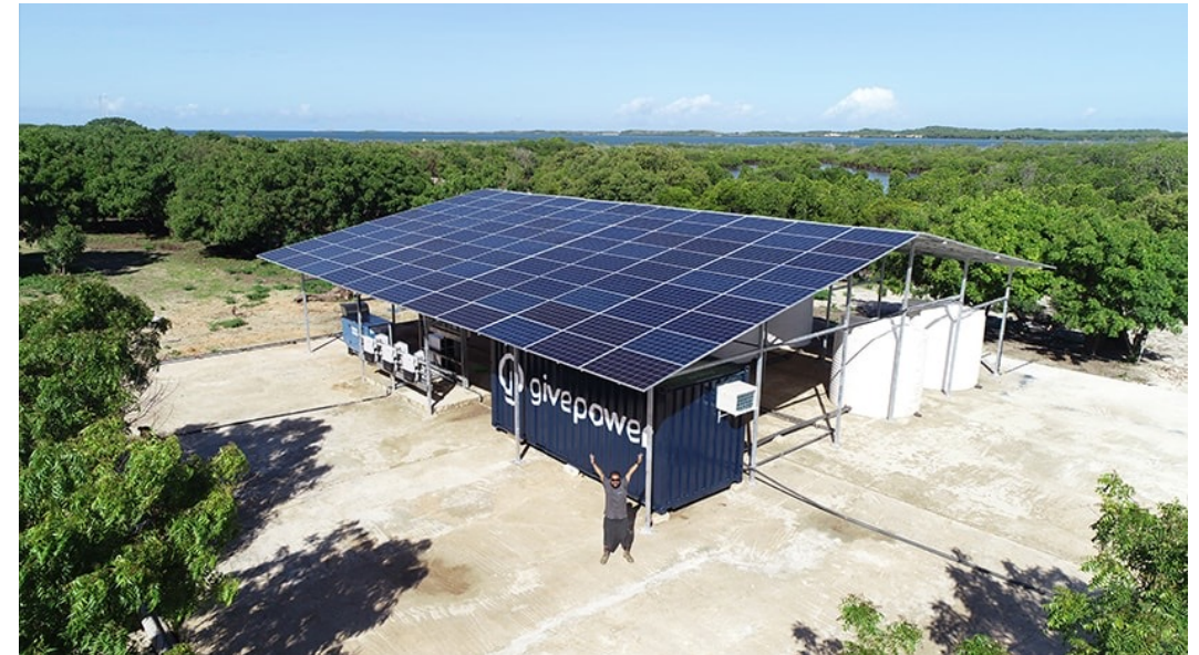
Example PV-powered RO Desalination Plant
